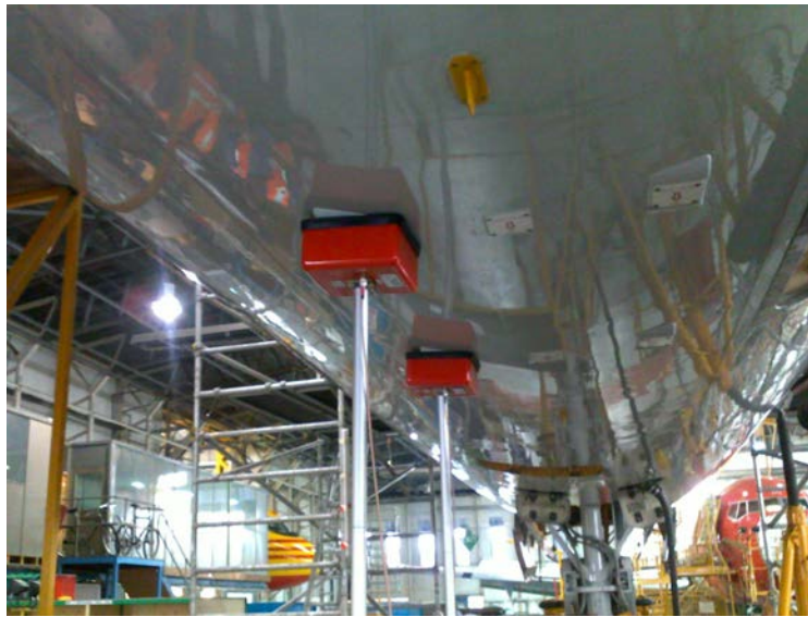
Fig. 4-14 ALT-9000 Antenna Coupler Installed
